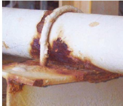
Above , the result of crevice corrosion on a pipe. Trapped moisture has caused substantial wall loss that could result in catastrophic failure.
